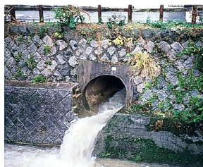
Photograph of the storm outfall from the combined sewer system during a heavy rain storm (Itabitsu River)
