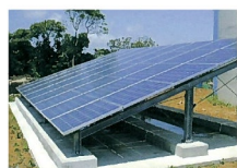
Ainoshima Solar Power Plant
