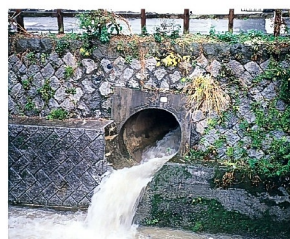
Photograph of the storm outfall from the combined sewer system during a heavy rain storm (Itabitsu River)
